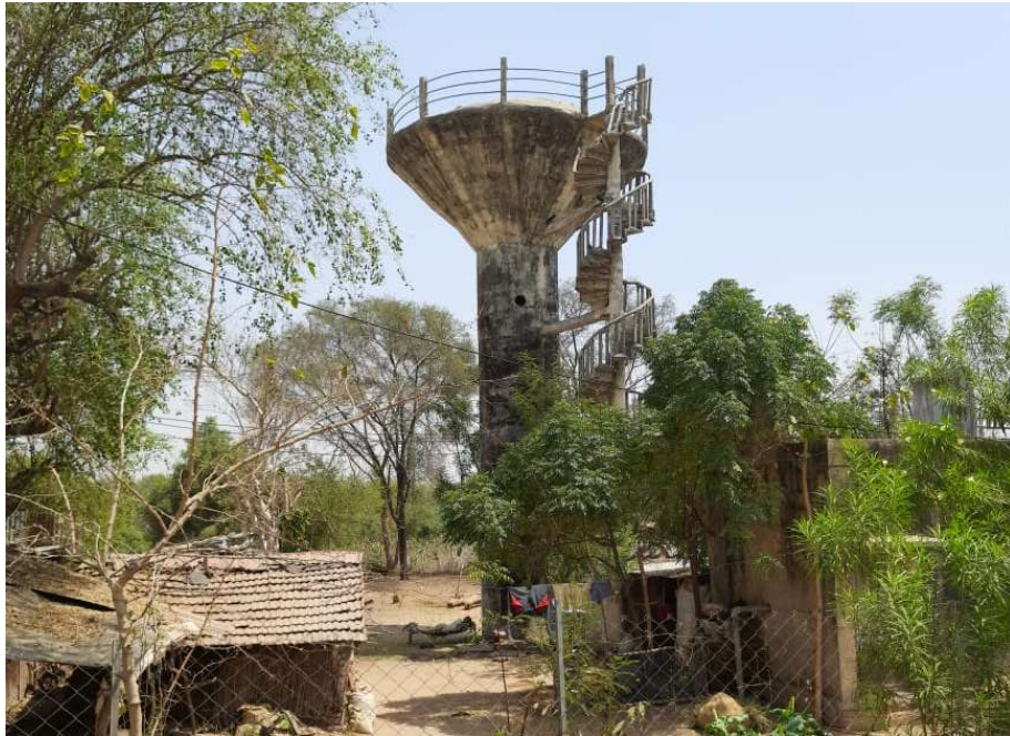
Photo 3.6: Abandoned Water Tank & RO System in Village
