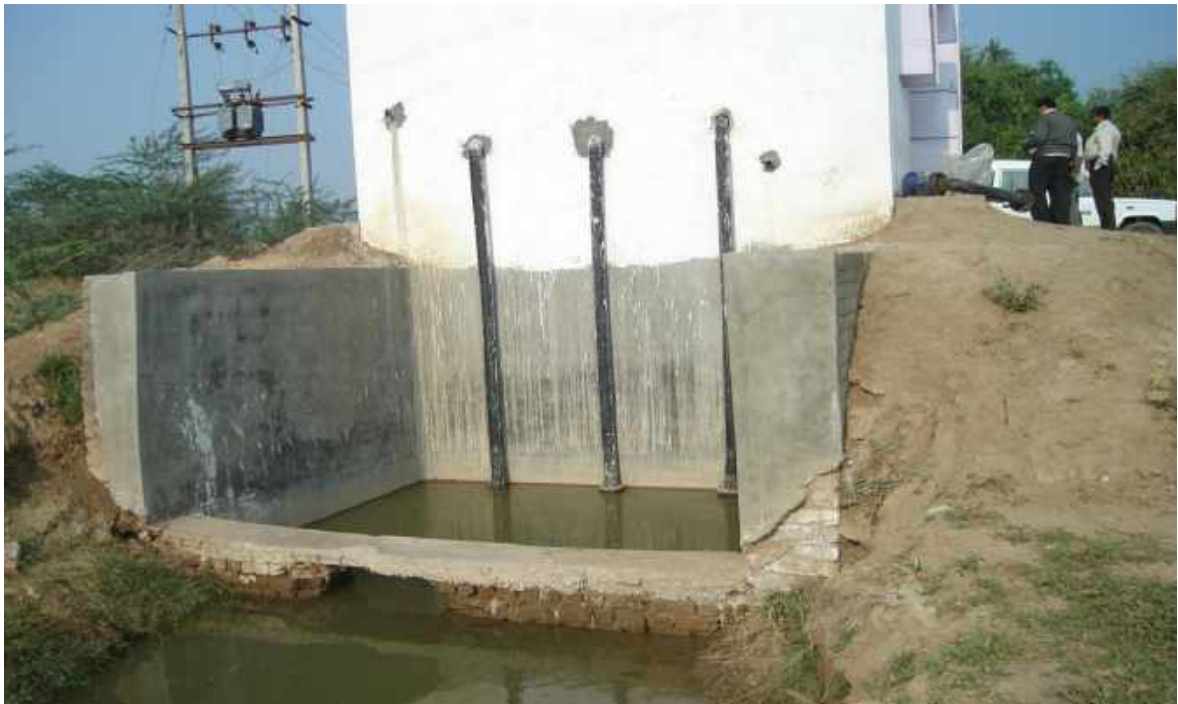
Figure 3.7: Intake Arrangement through Tank
